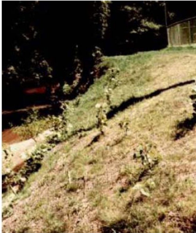
Figure 2: A stream bank six months after installation of mattress coir woven ECB.
