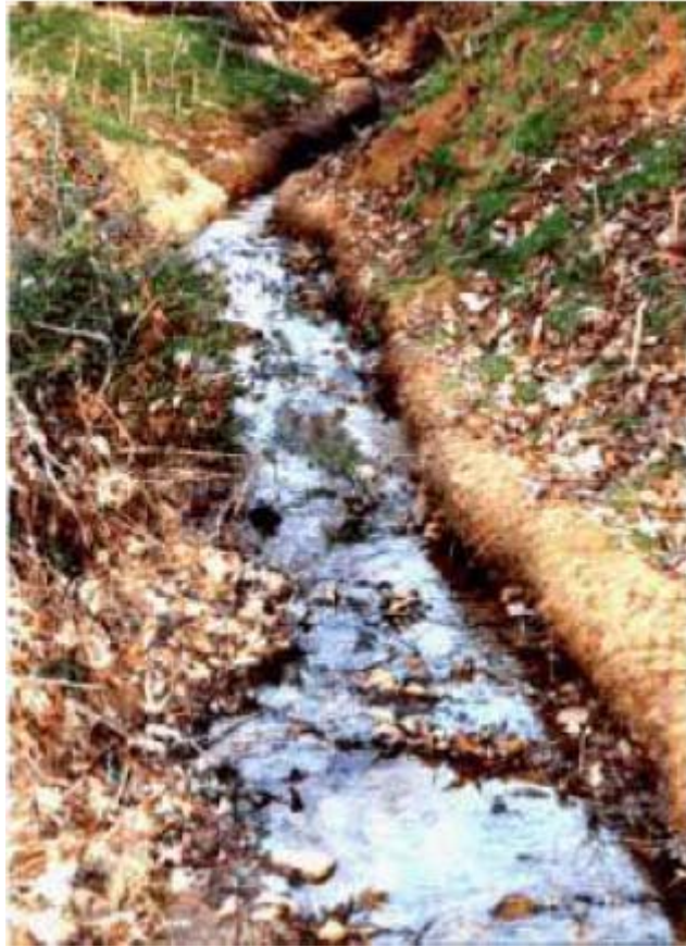
Figure 3: A stream restoration project one month after installation of mattress coir woven ECB and coir rolls.
